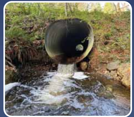
This impassable culvert under Hickox Road on Carpenter Creek will be removed and replaced with a bridge thanks to new grants.
